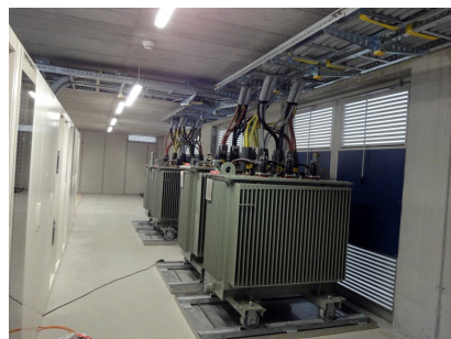
Blick in die neue Trafostation ...
