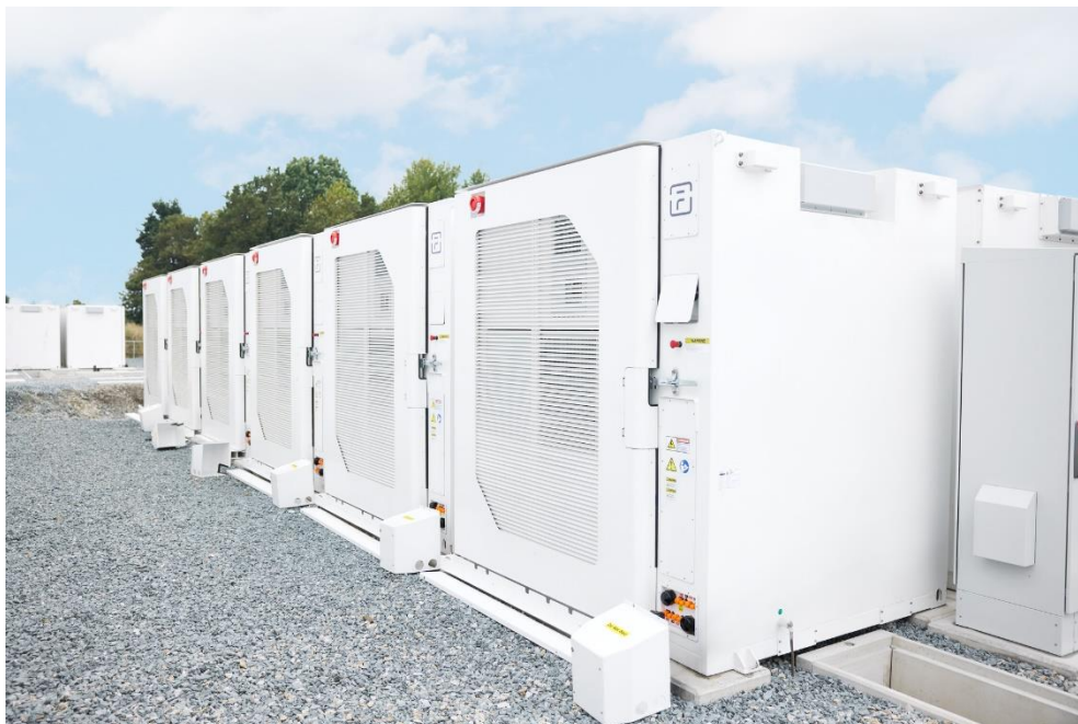
Batteries support the goal of a more flexible and sustainable energy system. (Illustrative image)
